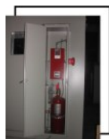
Fire Suppression System
